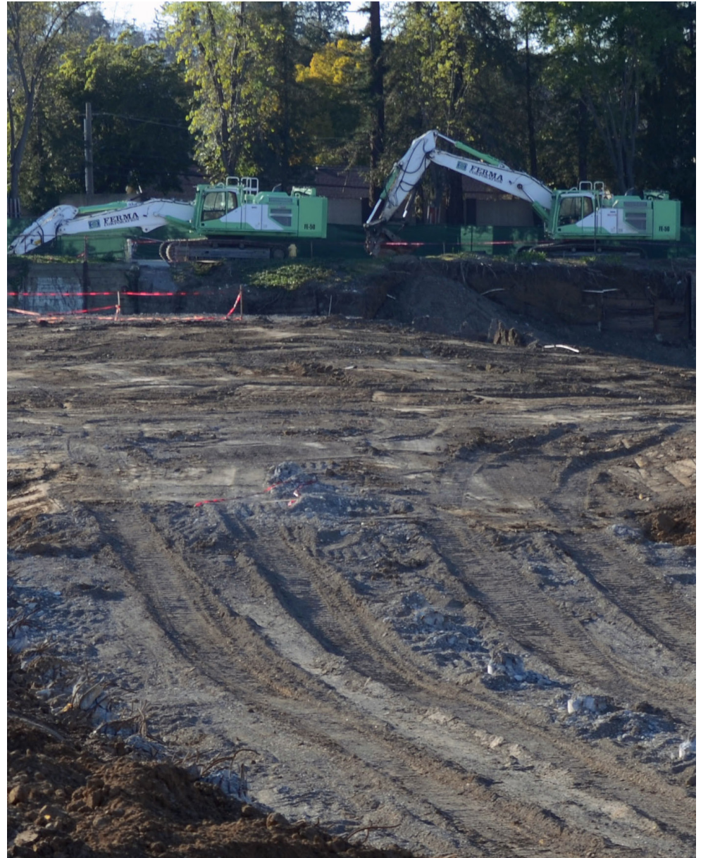
BULLDOZED Construction machinery digs up the parking lot of the former Vallco Shopping Mall in Cupertino. On May 7, a judge approved plans to convert Vallco into 2,402 housing units, half of which are below market-rate, and 1.8 million square feet of offices.
