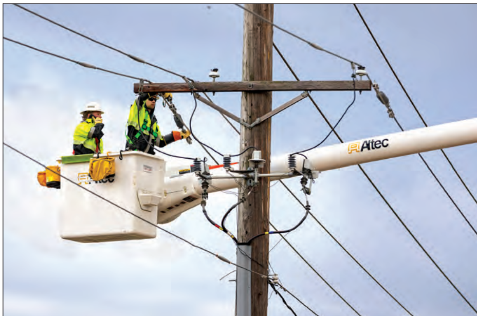
Ayrton Breckenridge/The Daily Iowan MidAmerican lineworkers fix electrical lines alongside Highway 6 after a tornado went through parts of Coralville on Friday. The Coralville fire and police departments worked alongside other agencies to help facilitate cleanup.
