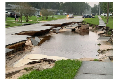
Collapsed street, Winter Springs
