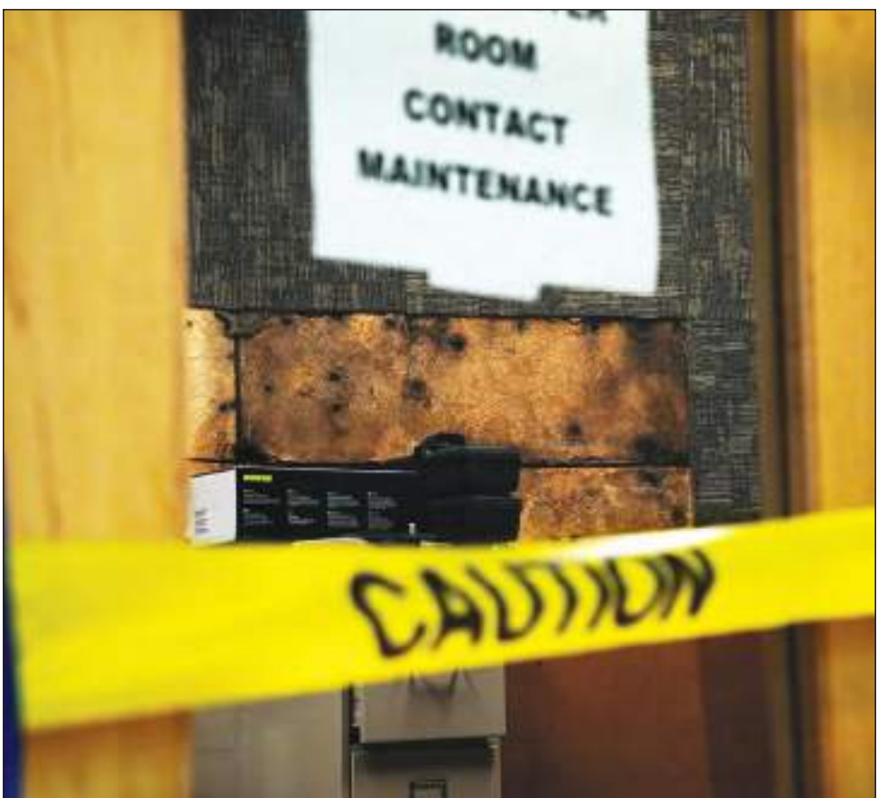
A view of the mold growing inside of Room 163D. This photo was taken Sept. 9.
